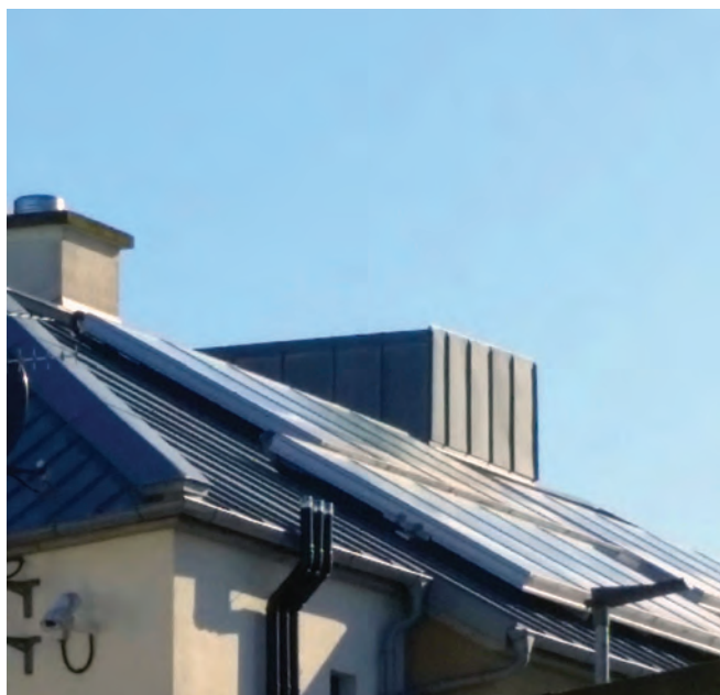
Photo: Solar thermal collectors on the rooftop
