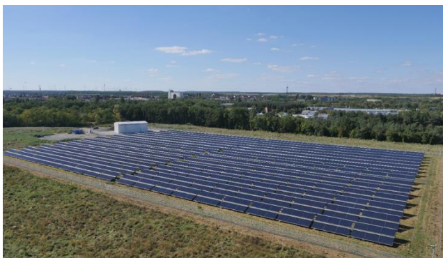
Figure 3: Exemplary 8300 m 2 evacuated tube collector system in Senftenberg, Germany. Source: Ritter Solar.
